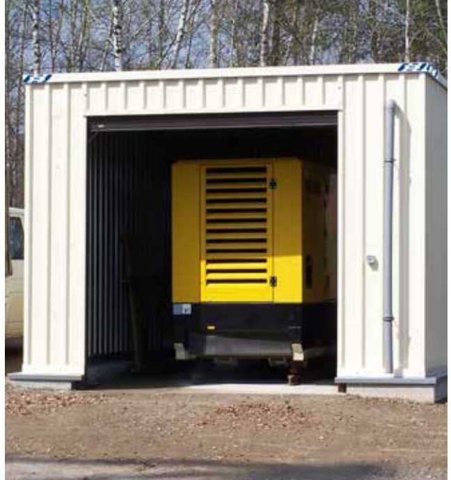
Power generator housing
