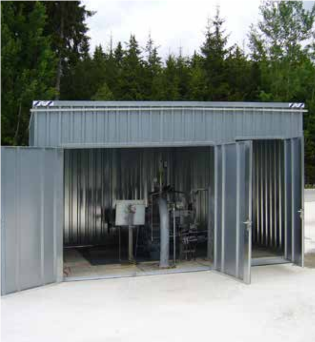
Gas pump housing
